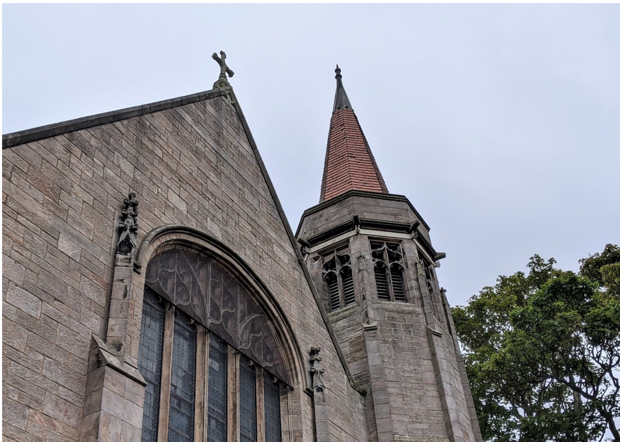
The west gable of Crail Community Hall – formerly St David's Church. (Source: Open Virtual Worlds / University of St Andrews.)
